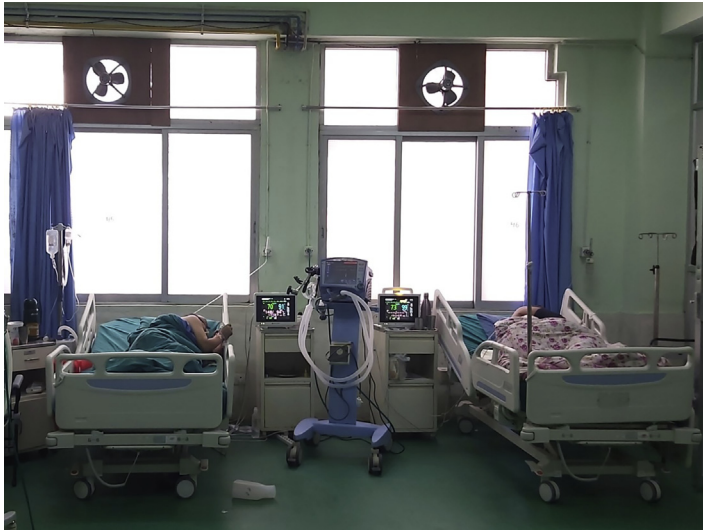
Fig. 1. Postanesthesia care unit is converted into COVID ICU. Because of lack of negative-pressure system, industrial exhaust fans were installed to minimize the viral load.
