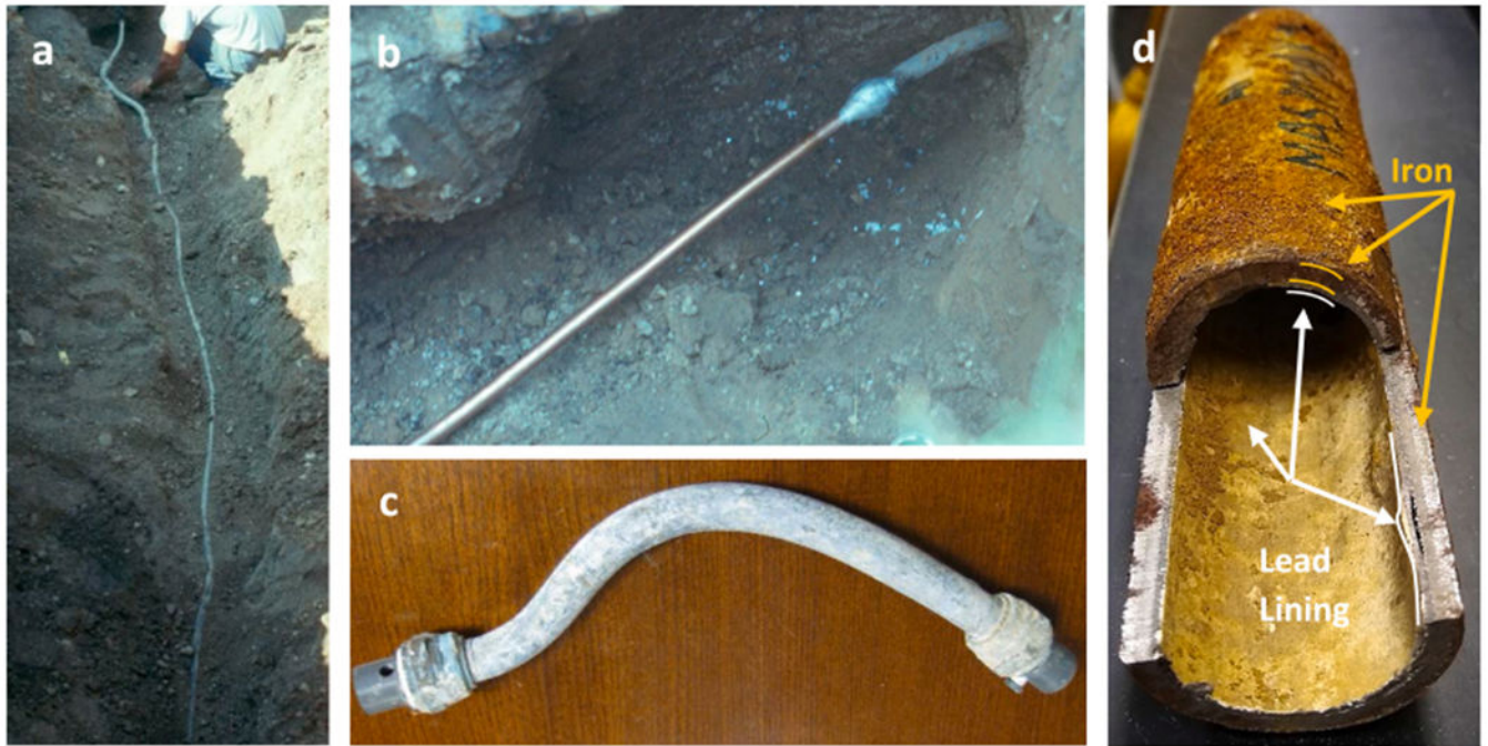
Fig. 3. (a) Full lead service line in the ground, (b) privately-owned lead service line partially replaced by copper pipe with a wiped solder joint in the ground, (c) lead gooseneck that was excavated, (d) lead-lined iron service line that was excavated and cut open to expose the lead-lining.
