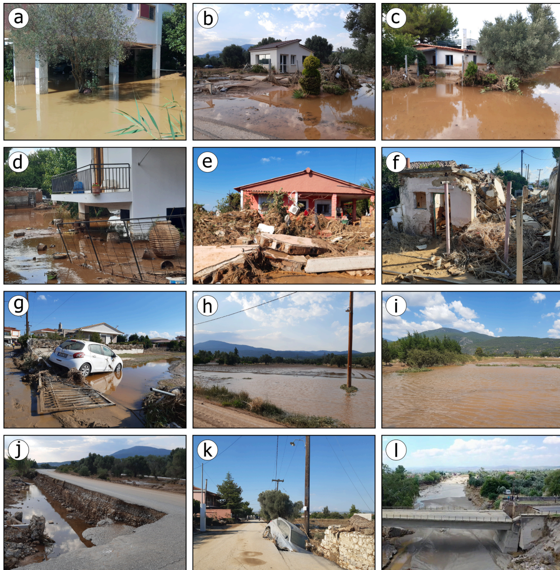
Fig. 7. Characteristic views of the flood effects in the Chalkida and Dirfia-Messapia municipalities in the Evia regional unit generated by the storm system Thalia. The induced floods resulted in damage to buildings including inundation of yards, basements and ground floors (a-d), damage to non-structural building elements (e) and damage to structural elements resulting partial collapse of the structure (f). Moreover, field crops were also affected by flood inundation (g-i). Damage to the road network included partial destruction of roads (j, k) and bridges (i).
