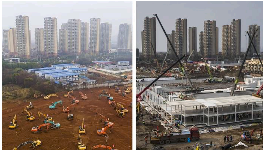
Fig. 9. Before (left) and after image (right) of the Huoshenshan Hospital in Wuhan, China [50].
