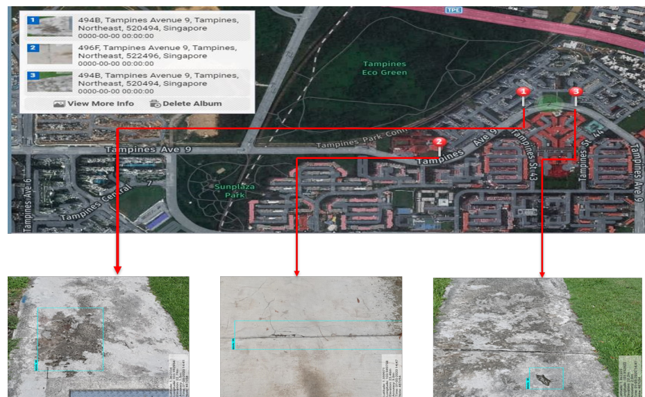
Figure 13. Defect location mapped on Google map.
