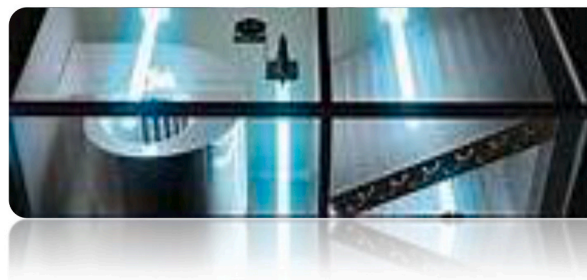
(e) Ultraviolet light bulbs in cooling coil
