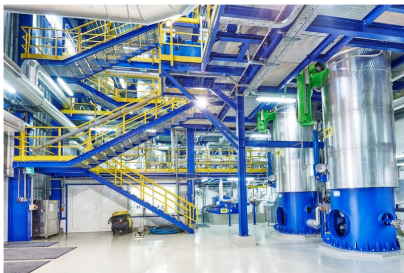
Figure 1. A modern industry plant of supercritical carbon dioxide extraction placed in Łukasiewicz Research Network—New Chemical Syntheses Institute (Puławy, Poland).
