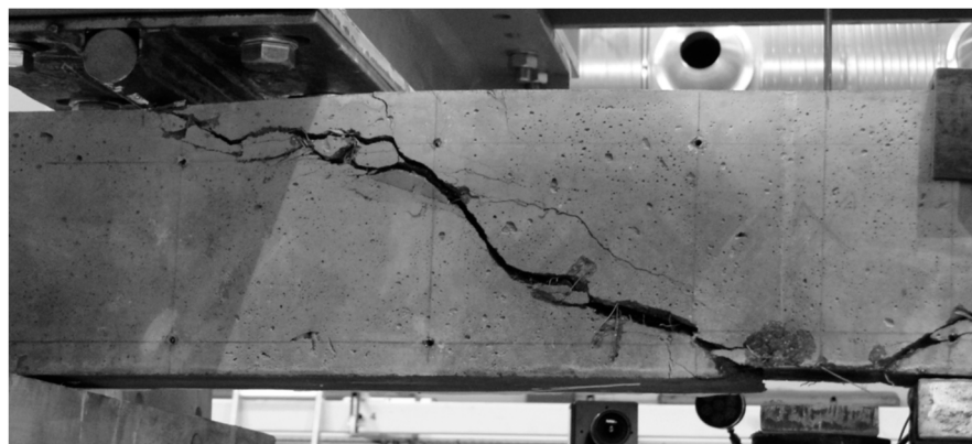
Figure 17. Example of a shear tension failure in the shear area of BF series beams.
