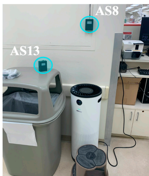
Figure 4. Photograph of the Surgically Clean Air Jade air purifier with three sensors (one sensor not in the field of view, located on the floor, in front of the air inlet of the filtration unit) to monitor the effects of the HEPA-filter-equipped air purifier.
