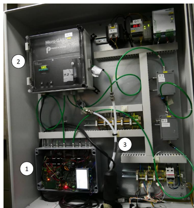
Figure 9. The internal components of the switch cabinet that were installed on the container ship PRIAMOS: (1) The developed photoacoustic SO 2 sensor system. (2) The MicroGASS gas sampling system (Perma Pure, LCC) dries and cools the gas sample down. (3) Gas inlet and outlet tubes of the measured gas from and to the switch cabinet, which pass through the temperature-controlled pipe.
