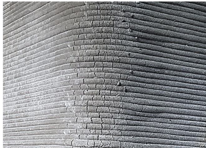
Figure 3. Development of cracks at the corner of a fresh-printed concrete wall.
