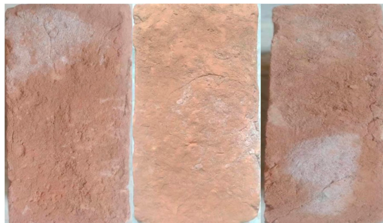
Figure 8. The effect of efflorescence.
