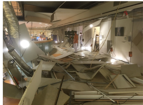
Fig. 1 Emergency department ceiling collapse due to construction failure
