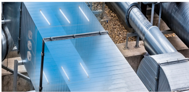
Fig. 43. In-Duct air disinfection system.
