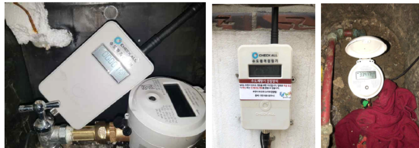
Figure 2. The left is the RWMR device installed in the household. The center is the AMI remote meter reader and the right is the water meter for remote meter reading.
