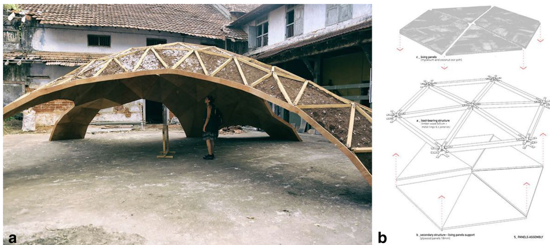
Fig. 4 a Exterior Perspective of the pavilion. Credit: © Krishna and Govind Raja. b Exploded diagram of the different construction layers. Credit: © BEETLES 3.3—Yassin Areddia Designs
