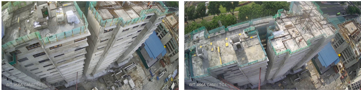
Fig. 6. Snapshot of CCTV camera system.
