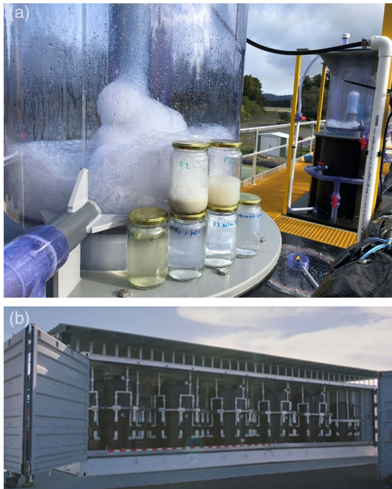
FIGURE 3. (a) Foam fractionation column treating PFAS-laden water (photo courtesy of Evocra Pty Ltd). (b) Foam fractionation system (photo courtesy of OPEC systems and Dora Chiang, CDM Smith)
