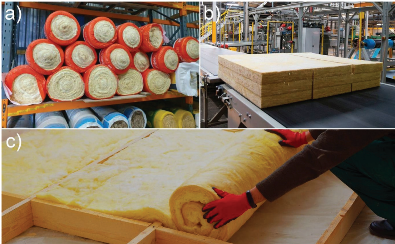
Figure 4. a) Packaged rolls of glass MWI. b) Cut slabs of glass MWI prior to packaging. c) An installer unrolling a MWI product at a construction site.
