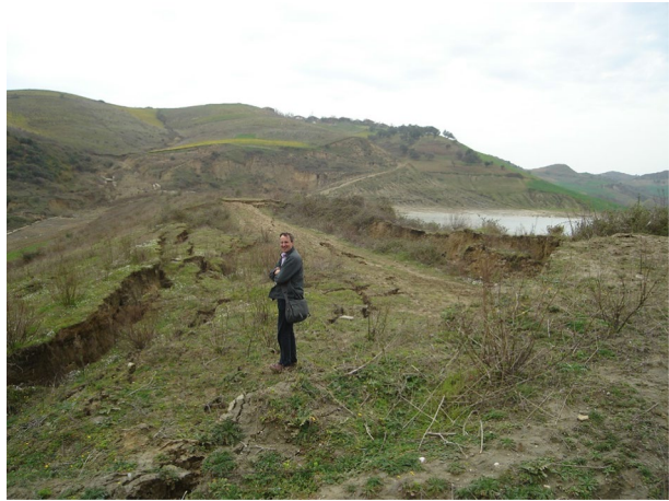
Fig. 113 Damage to the Sharredushk dam caused by an earthquake of M 4.1 (Courtesy of Mr Tim Hill)
