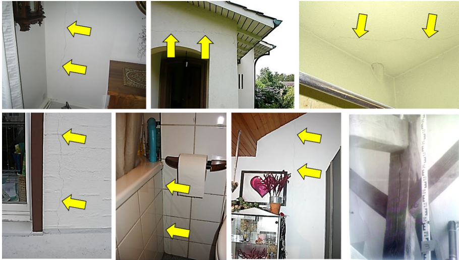
Fig. 120 Examples of reported earthquake damage caused by the M_L 3.4 Basel earthquake (Courtesy of Geothermal Explorers); in each case, the yellow arrow highlights the crack, except in the bottom right-hand image, where the ‘damage’ is splitting of timber due to drying
