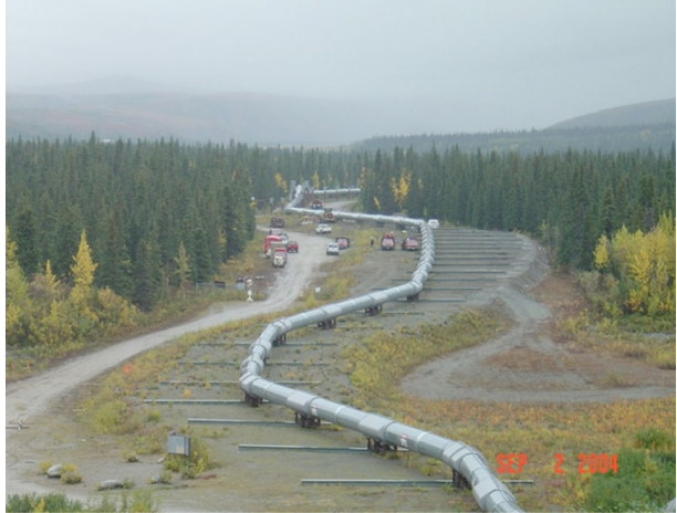
Fig. 10 The Trans-Alaska pipeline crossing of the Denali fault, restored to its original configuration following the 2003 Denali earthquake to be able to withstand right-lateral displacement in future earthquakes (Image courtesy of Lloyd S Cluff)
