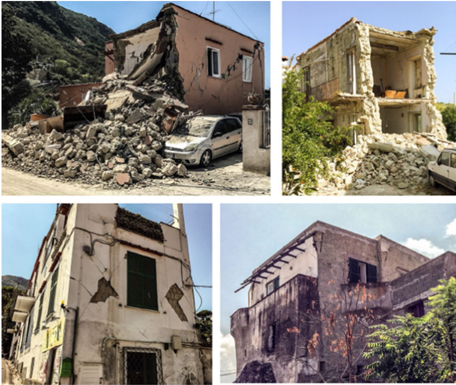
Fig. 107 Upper and lower left: Examples of damage to unreinforced masonry buildings in the 2017 M 3.9 Ischia earthquake; lower right: undamaged masonry building with iron tie rods (Brishghella et al. 2019)
