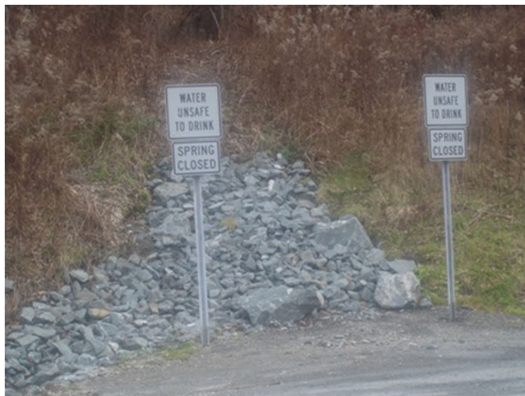
Fig. 2. Roadside spring box demolished, located on Route 22 in the town of Stephentown, Rensselaer County, New York.
