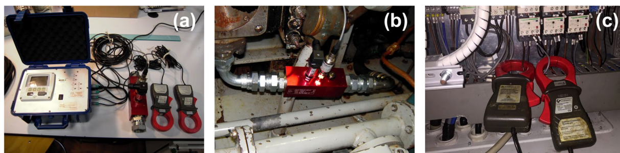
Fig. 5 AC electric and hydraulic data collection system. (a) Complete system; (b) hydraulic sensor measuring the flow and pressure from the hydraulic pipeline; and (c) clamp-on ammeters measuring the electric power supply from the alternator.
