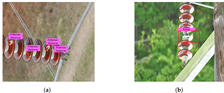
Figure 1. Two different types of defects: (a) pollution flashover; (b) damage.
