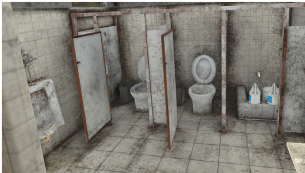
Figure 8. Level 2 of dirtiness in bathroom.
