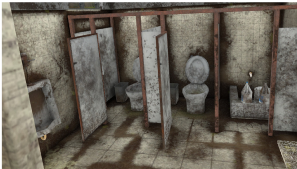
Figure 9. Level 3 of dirtiness in bathroom.
