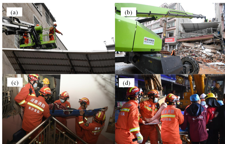
Figure 4. (a,b) Rescuers perform rescue operations; (c,d) Rescue work by relevant personnel.
