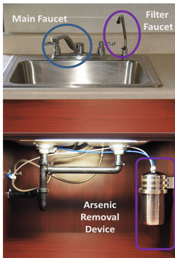
Figure 1. Filter device, showing POU arsenic filter installed under kitchen sinks and filter faucet.
