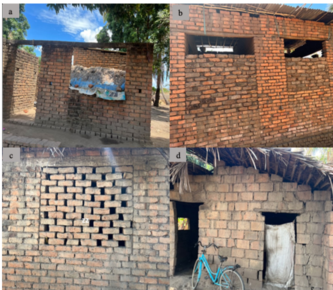
Fig. 4 Examples of improved but incomplete houses that people were residing in: a un-roofed house, b bricks on windows with small gaps on top, c holes in the walls and d no door covers, open eaves
