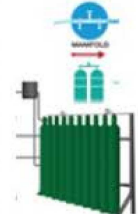
Manifold (filling and/or distribution ramp)
