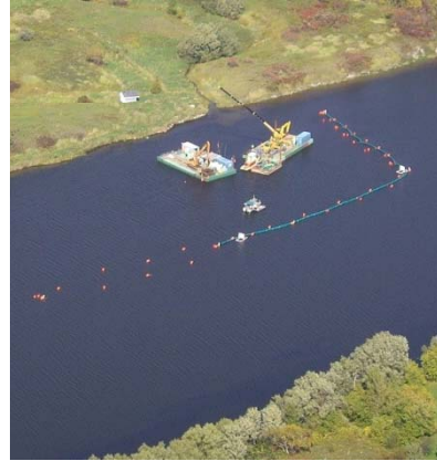
b) Application of activated carbon under 15 feet of water at Grasse River, NY, USA (2006). The site was enclosed with a silt curtain and application was performed using a barge mounted crane. Placement and mixing of the AC was achieved using two devices: 1) a 7-by-12-foot rototiller-type mixing unit; and 2) a 7-by-10-foot tine sled device.
