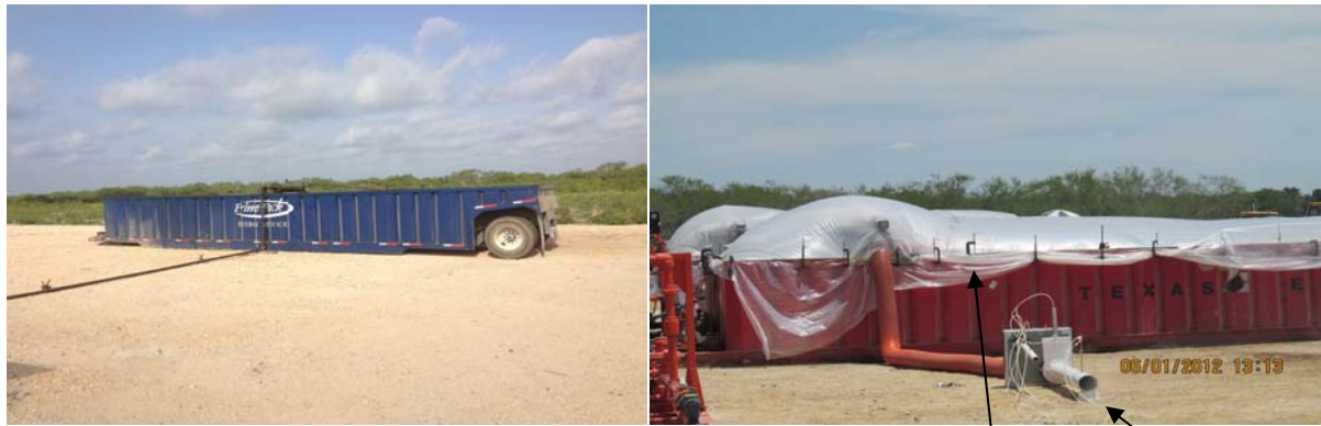
Figure S1-2. Open top tank used in Step 1 of flowback using the equipment configuration shown in Figure S1-1. Upper Left: line leading from well to tank; upper right: temporary plastic cover installed and clamped to edge of tank, with exhaust stacks on ground adjacent to tank; lower: Conceptual diagram of sampling system.
