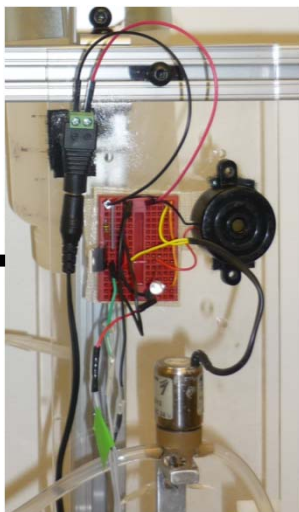
20-V solenoid valve circuit and water reservoir
