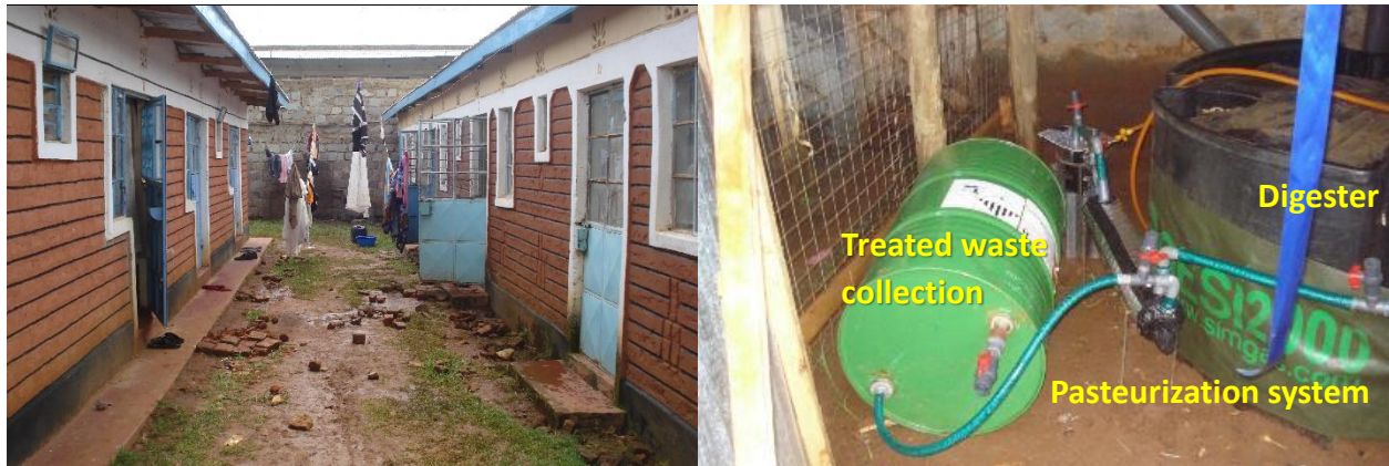
Figure S2. Layout of Central (top), view of the plot looking towards the location the ADPL was installed (bottom, left) and view of the treatment system enclosed below the latrines superstructure (bottom, right).
