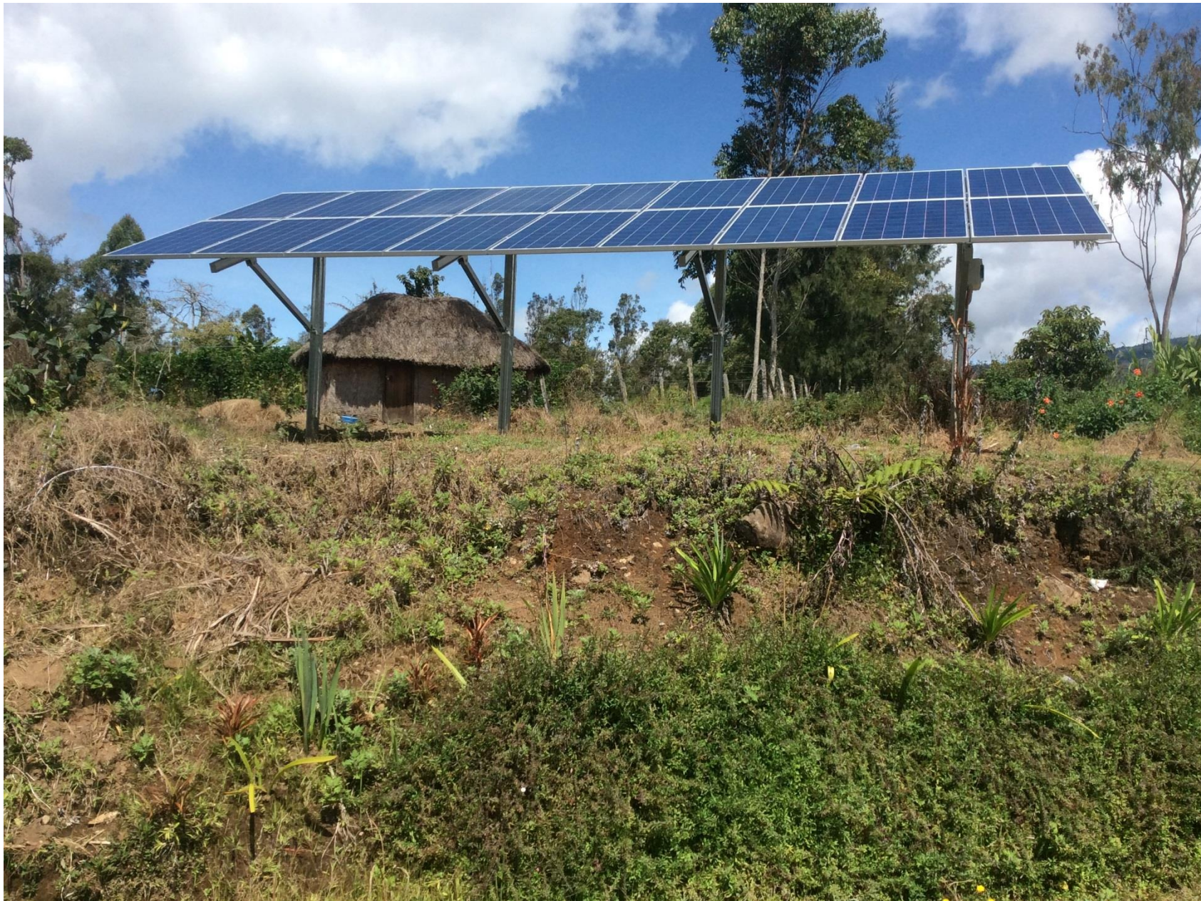
Solar panel configuration at Keripia Health Centre, Western Highlands Province, PNG
