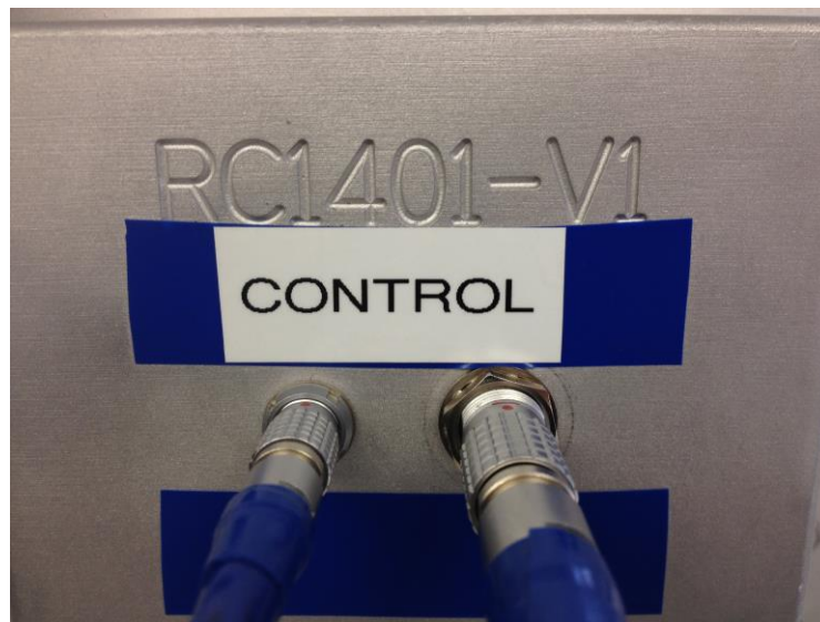
Pictured above: Connectors from the cart plugged into the filter box. Note the matching colors of the cables and box.
