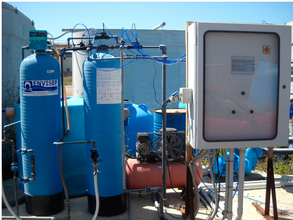
Figure S9. Picture of the pilot plant.
