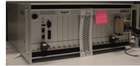
Photo of digital control system
