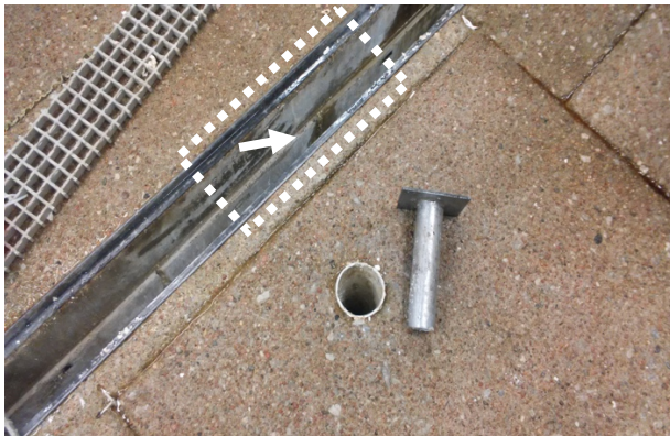
C. Trench drain with grate removed and cleanout opened (B8, B9, B10, B11).
