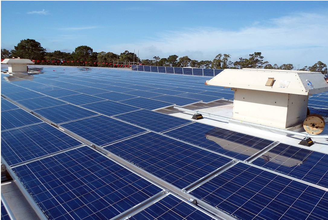
Image from Wikimedia Commons: By U.S. Army Corps of Engineers Sacramento District - Solar panels at Presidio of Monterey, Public Domain, https://commons.wikimedia.org/w/index.php?curid=52215100
