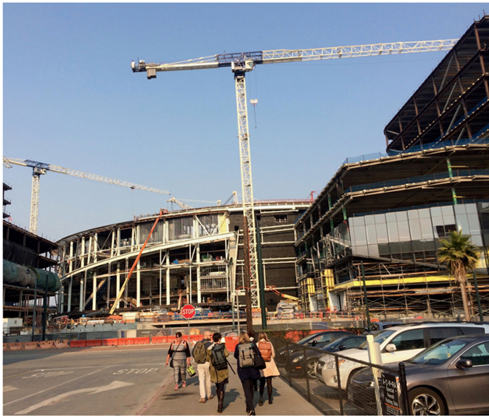
Figure 2. Research team members lead a walking tour in Mission Bay. Visible in the background is the construction of the Chase Center, future home of the Golden State Warriors. Photo credit: the authors.
